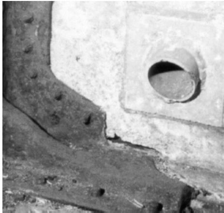
Figure 10.10: Bi-metallic corrosion. The aluminum and steel are in contact in the presence of water and dirt. The aluminum corrodes, forming aluminum hydroxide. The steel is protected from corrosion.
